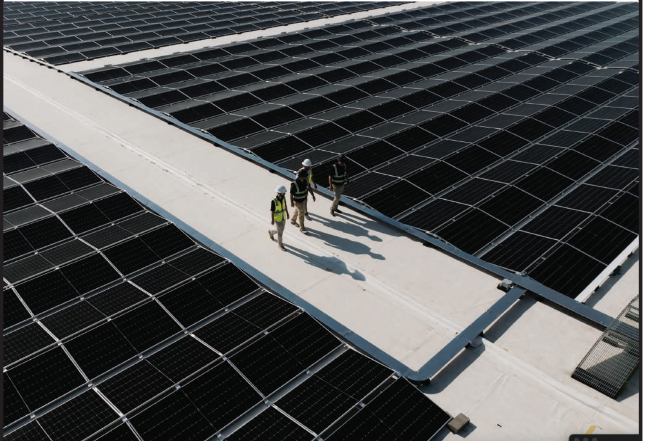
Workers from Primus Builders ( No. 278 ) survey the installation of a 1-MW solar array on the roof of a 295,000-sq-ft greenfield cold storage warehouse in Ridgeville, S.C., which will produce 1.5 million kwh of energy. On track to achieve LEED Gold certification, the facility will also feature a 50,000-gal rainwater capture tank to be used as part of an adiabatic cooling system that reduces the water requirement by 50% compared to traditional cooling tower systems, Primus says. Materials have been sourced regionally, and had their Environmental Product Declaration reviewed to make sure no ingredients were on the red list.
