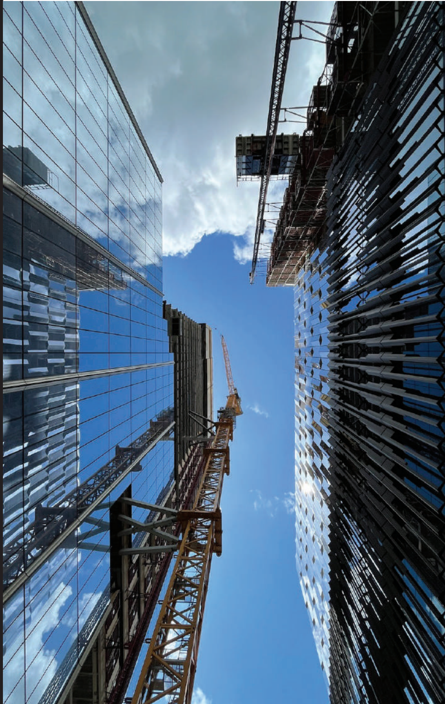
Barton Malow ( No. 19 ) recently topped out Hudson's Detroit, a 1.5 million-sq-ft, 685-ft high mixed-use development in the city's downtown. The project is located on the former site of the J.L. Hudson department store, one of the largest U.S. retail stores before its controlled demolition in 1998. The replacement structure will be Detroit's first skyscraper in 30 years, Barton Malow says. More than 2.7 million worker hours have gone into the project.
